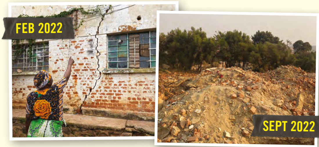
© ↑ Cécile Isaka showing crack in her house caused by the activities of the Kolwezi copper and cobalt mine operated by COMMUS, February 2022 (left); Ruins of Cécile Isaka’s house, September 2022 (right) © Amnesty International (photographer: Jean-Mobert Senga)
