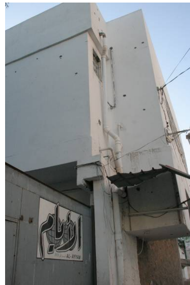
al-Ayyam building damaged by bullets © Amnesty International
