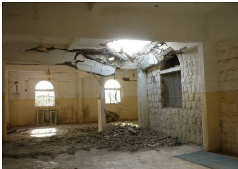
Inside a building that took a direct hit, Sa'dah, Yemen, March 2010 © Private
