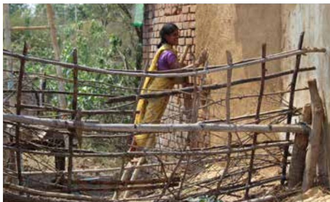
A woman plasters the walls of her house in Sonpuri village, April 2014. © Amnesty International India
