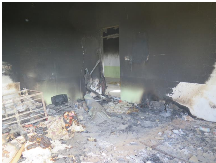
Jiri – inside a burned house, all the rooms were similarly destroyed © Amnesty International
