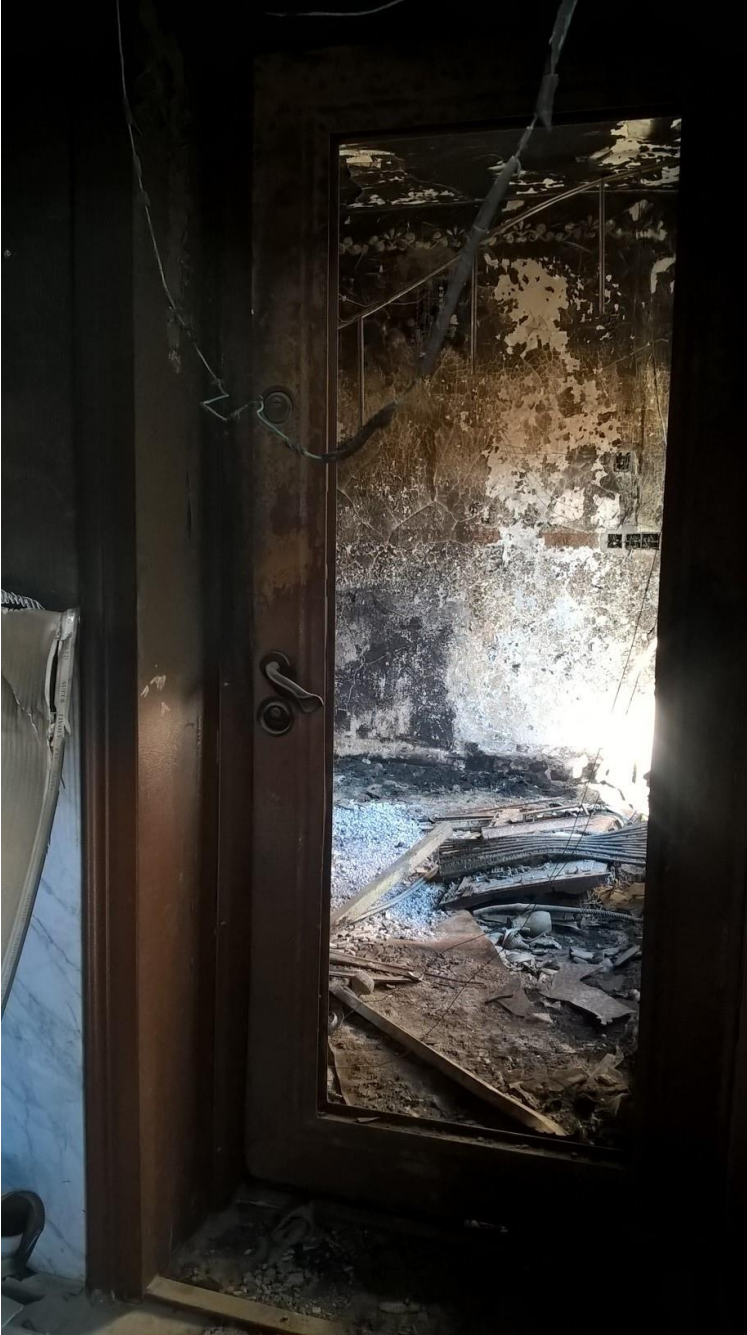
Burned house in Makhmur © Amnesty International
