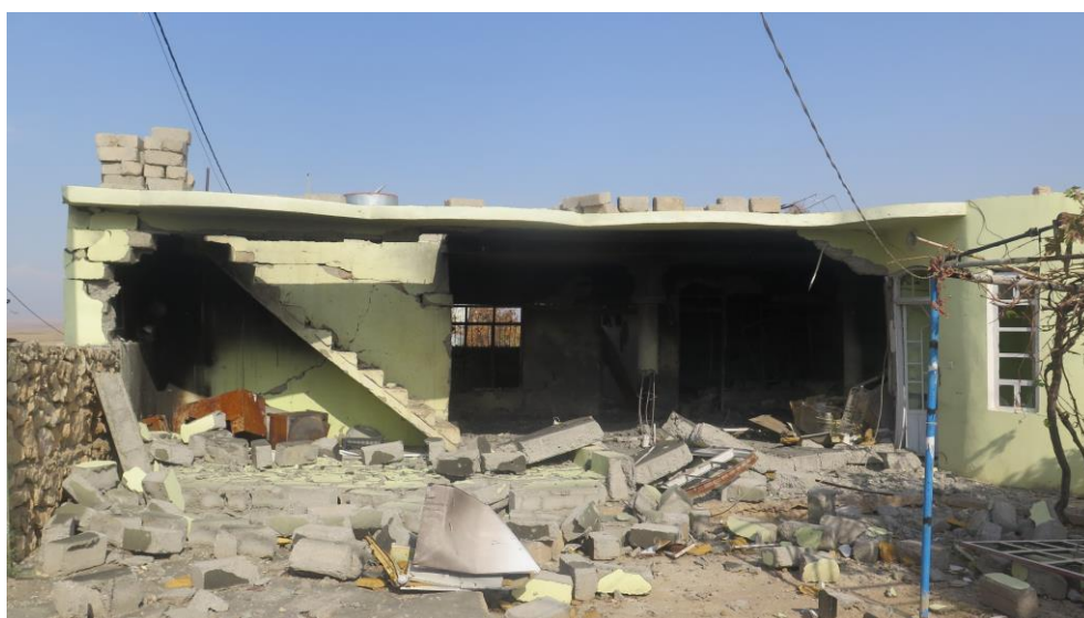
Destroyed house in Barzanke © Amnesty International
