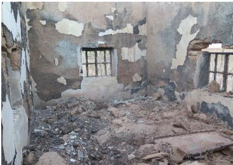
A room destroyed by fire in the home of Bassma Mohamed al-Bilal in Tel Diyab. © Amnesty International
